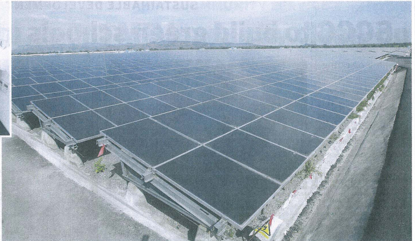
NED'S SOLAR farm in Lop Buri is now producing power to the Electricity Generating Authority of Thailand.
