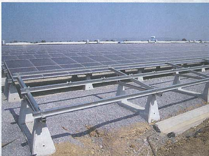
THE 1,200-RAI plant will use 540,000 solar panels to produce 84 megawatts.
